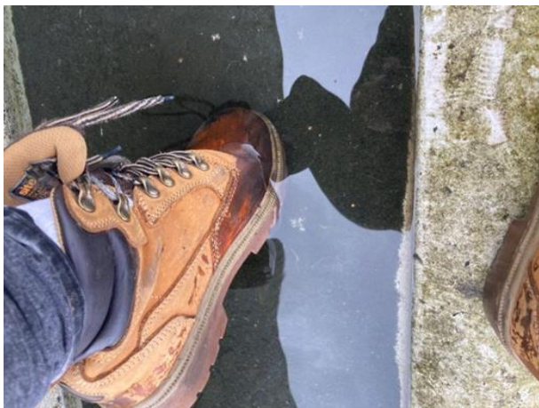
Further evidence of major ponding inside the gutter.
