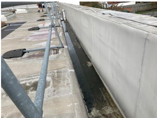
Overview of gutter with ponding inside
