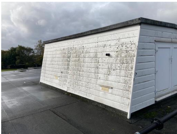
Tank room with UPVC cladding
