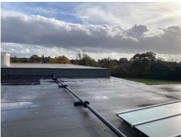
Pipe work on supports present on the roof
