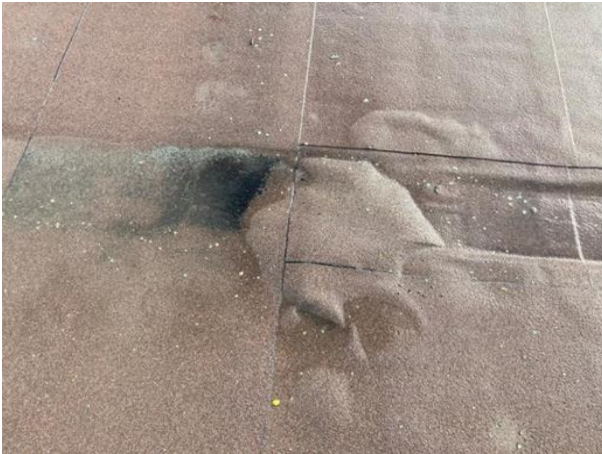
Evidence of blistering on the roof.
