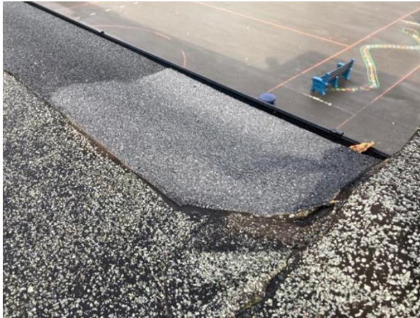
Evidence of previous repairs
