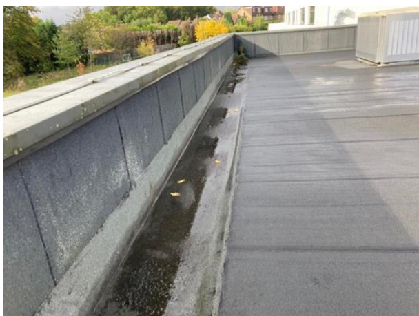
Overview of the gutter with evidence of ponding
