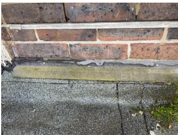
Mastic repair to the upstand indicating previous water ingress issues.
