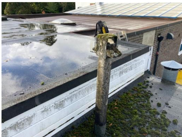
Possible ACM soil vent pipe present on the roof.
