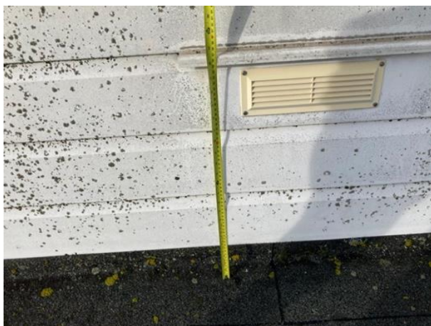
Wall cladding 120mm above the roof surface. Wall vent circa 450mm above the roof surface.
