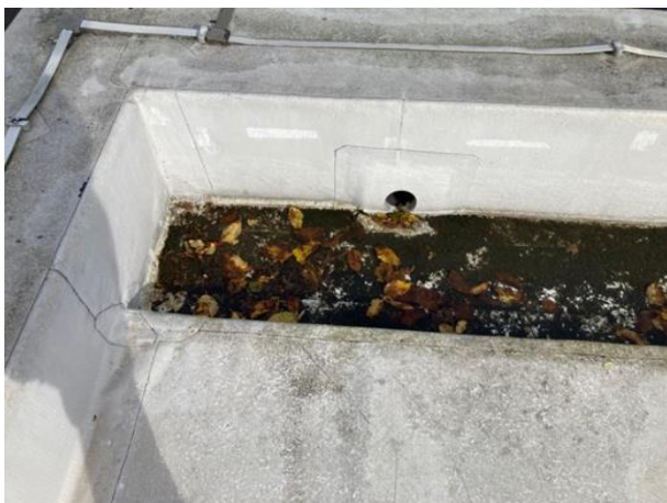
Internal gutter with evidence of ponding water
