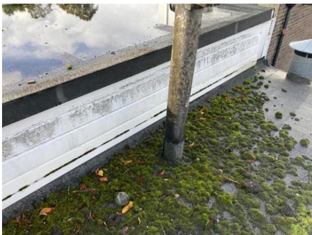
Moss growth present on the roof
