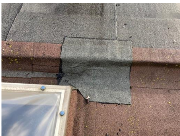
Evidence of previous repairs
