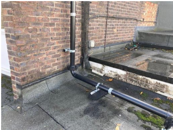
Overview of Roof B Pipe work with support present on the roof
