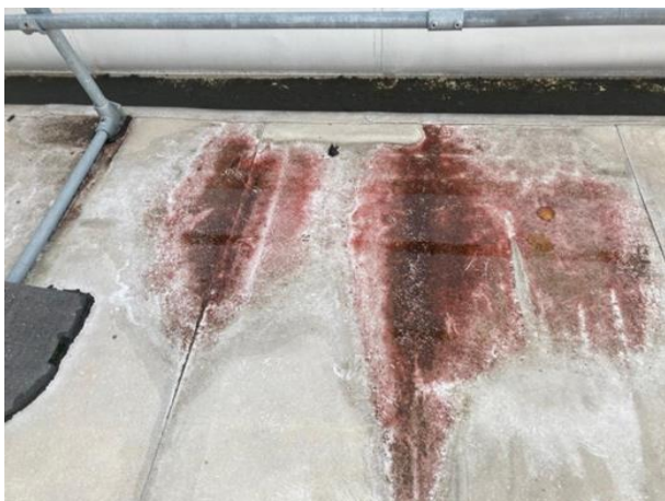
Evidence of failing single ply
