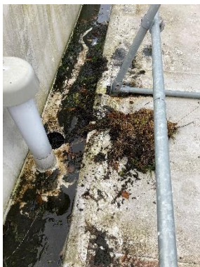
Partially Blocked (Cleared some but needs further work)
