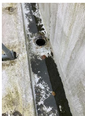
Drain higher than surrounding roof channel leading to permanent standing water
