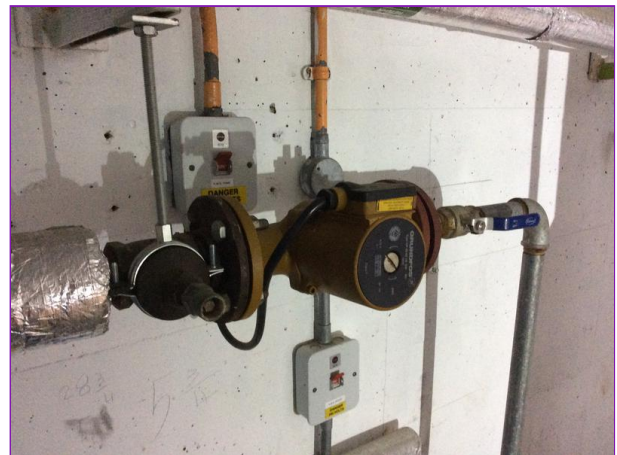
Photo 370 - East block original school HWS circ pump
