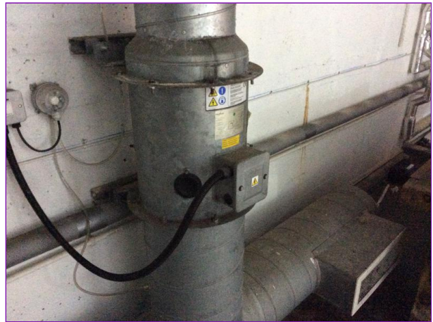
Photo 372 - East block original school plantroom vent fan
